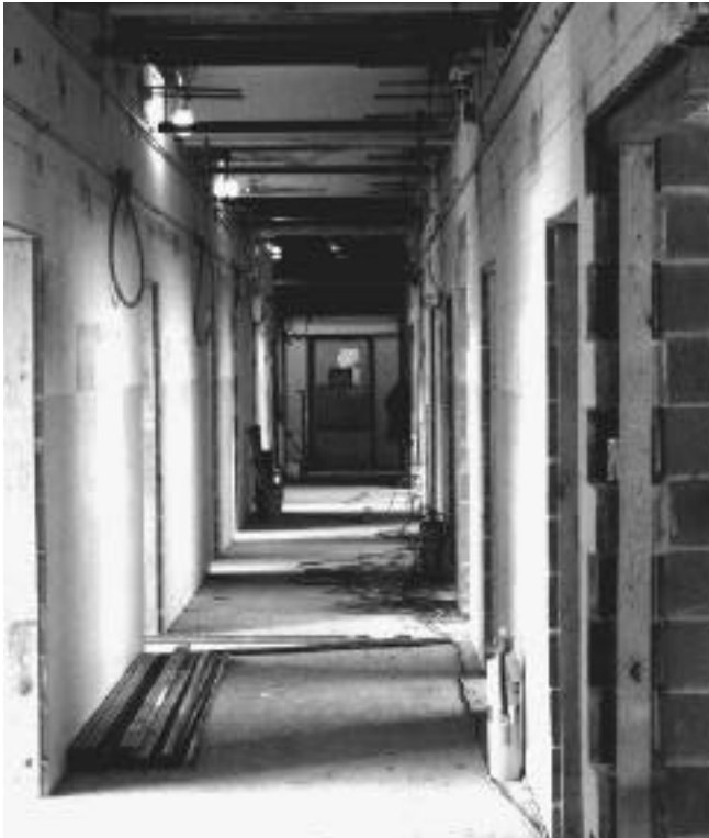
A typical view of a hallway under renovation. While this work was going on in one part of a building, state-of-the-art optics research was being carried on in another part of the building.
