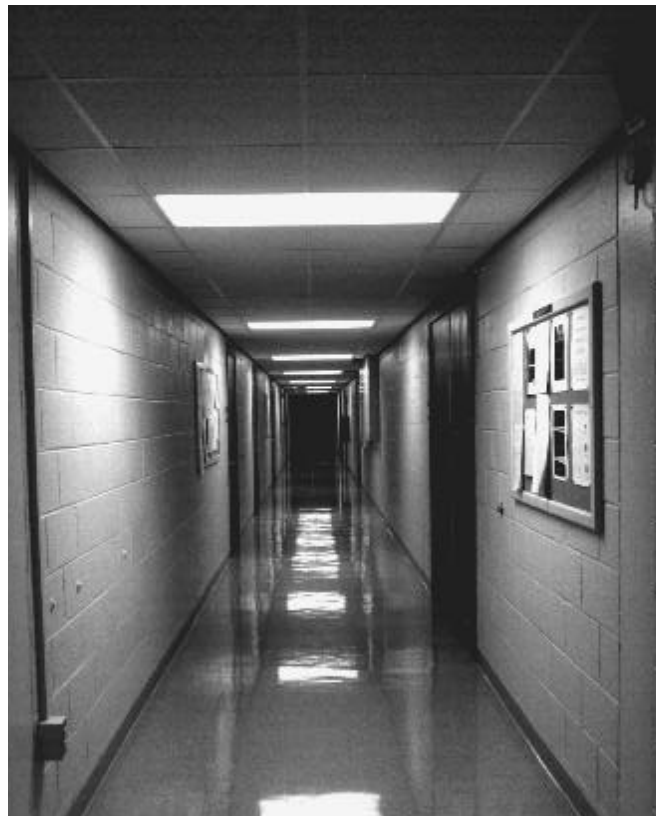
East hallway on the ground floor of the Building after renovation. The same hallway before the renovation is shown on page 140.
