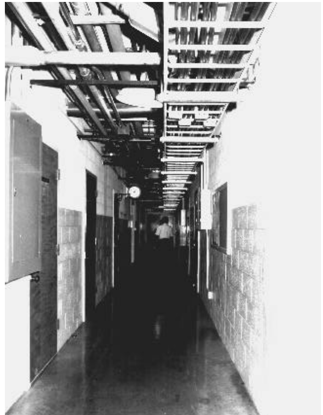
A view of the east hallway on the ground floor. The hallways had exposed utilities and were dimly lit by incandescent lights.
